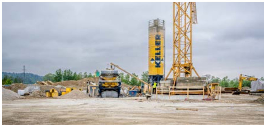
CENTRAL CORRECTIONAL FACILITIES PROJECT IN LJUBLJANA in the final stage of implementing ground improvement works with VMCs.
