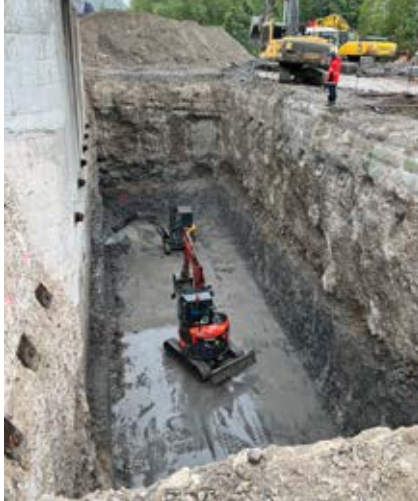
DIGGING OF THE CONSTRUCTION PIT for the P1 pillar. You can clearly see the difference between the individual geological layers.
