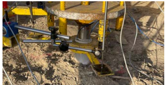
FIBRE-OPTIC SENSOR CABLES (BLUE) IN THE PILE, along with displacement transducers during the test execution
